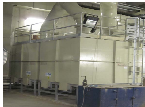
Parallel Bed Scrubber (PBS)
